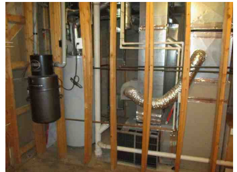
Central Vacuum / Furnace
