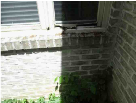
Damaged Window Frame
