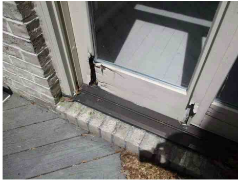
Damaged Window Frame
