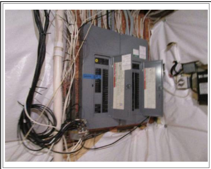
Basement - Electric Panel
