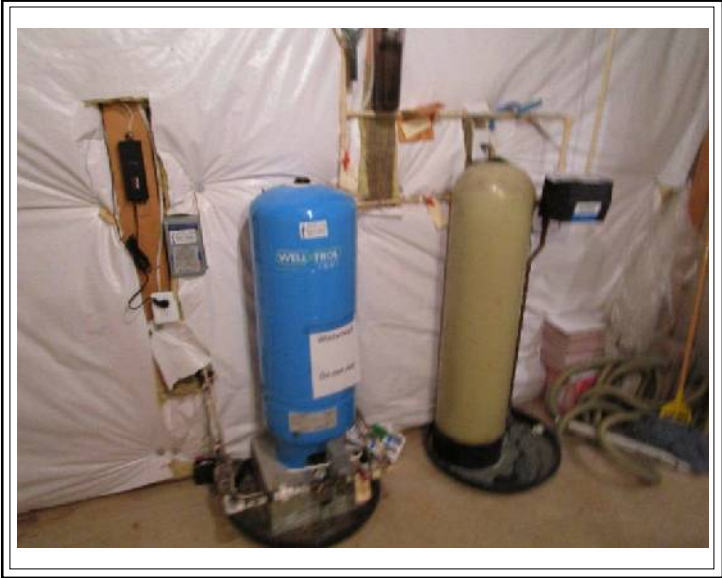
Basement - Well Equipment
