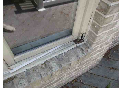
Damaged Window Frame
